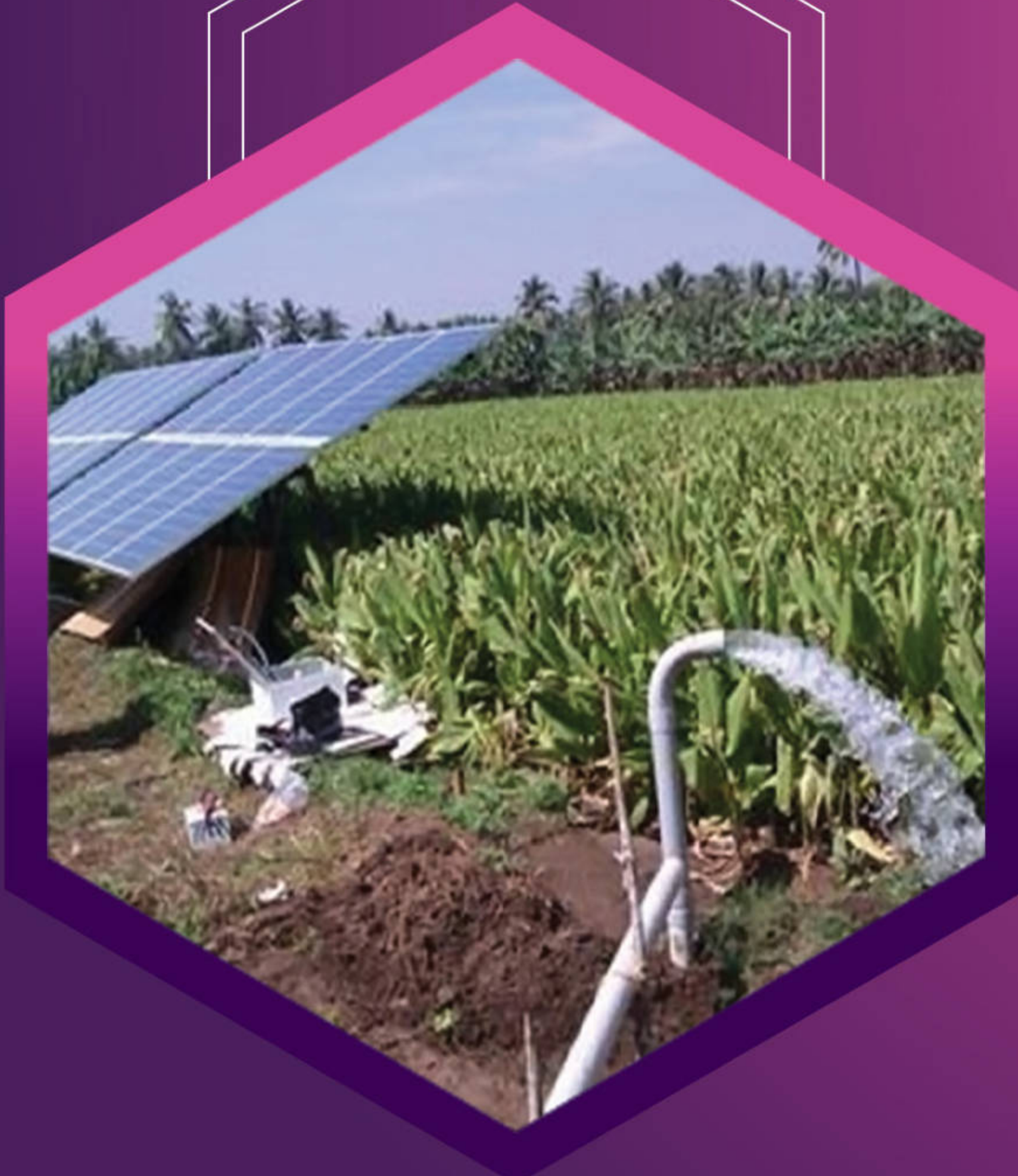
Solar Irrigation Pump System
